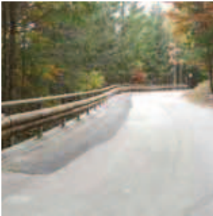
Two half round log diameter 22 cm, length 4.00 m backed with a steel U profile
